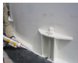
Tank Chime Sealant
